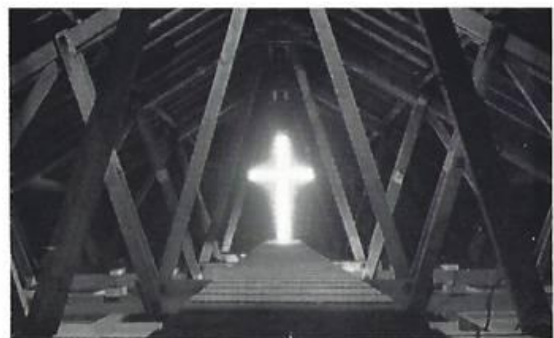
A VIEW OF THE ROOF TIMBERS, TAKEN ABOVE CEILING LEVEL, ILLUMINATED BY THE GLASS CROSS IN THE FRONT GABLE
